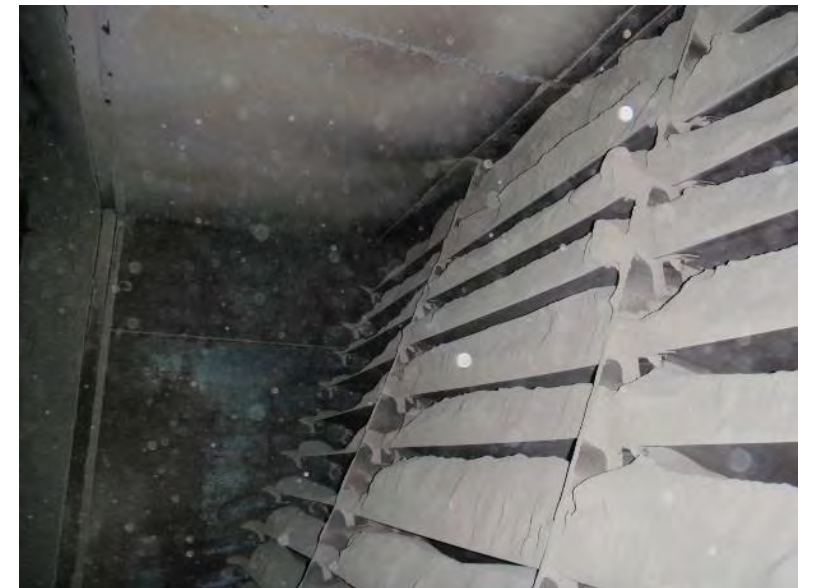
Inlet screen partially blocked
